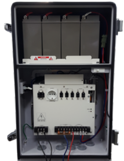
Portero 30A Inside (with batteries)
