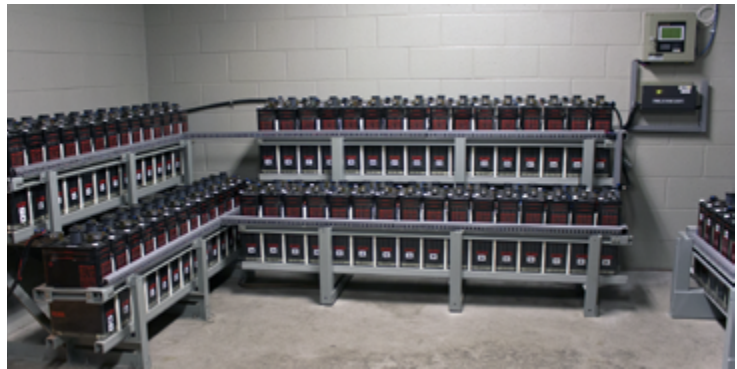
iPQMS Installation on 125VDC Utility Battery System
