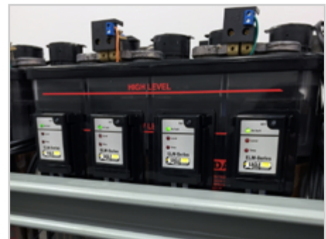
Electrolyte Level Sensors Installed on VLA Utility Battery
